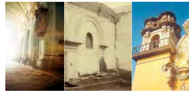
Fig.4 The Compañía Church, Pisco: a) Adobe walls with humidity and differential settlement; b) Adobe walls with loss of the original locking elements and the ties between themselves; c) Crack separating the walls of the tower and façade of the nave (credits: Pedro Hurtado Valdez, 2007)
