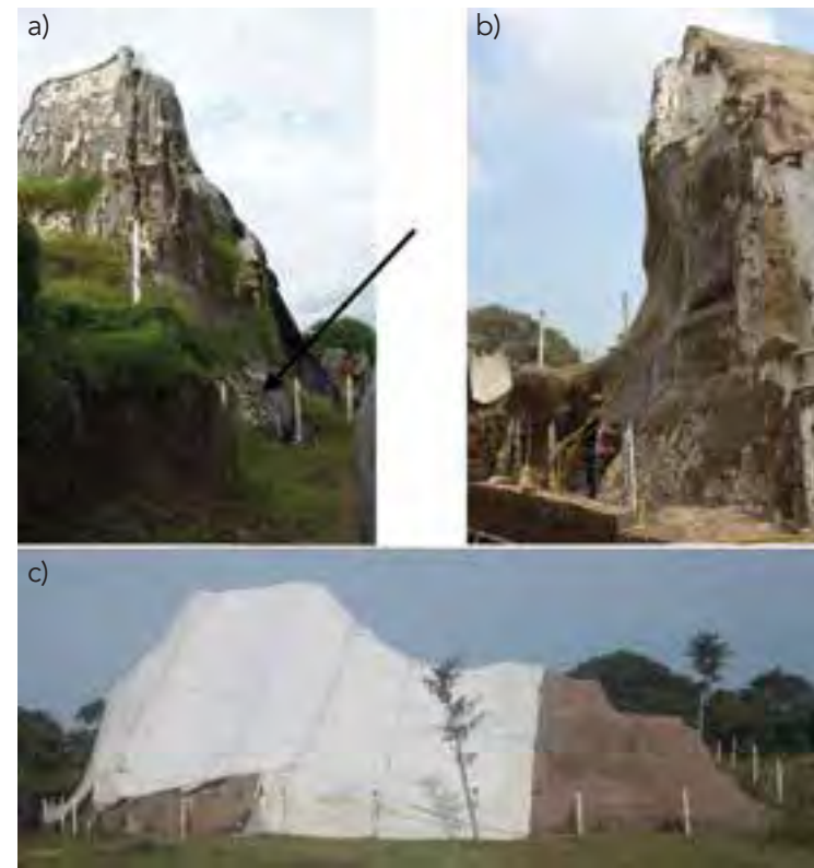
Fig.4 La Joya Pyramid in spring 2010: a. arrow indicates collapse of north retaining wall due to weeds, b. geotextile applied directly to north profile, c. west façade protected by tarpaulins, whereas for the southern sector (on the right) with the new sacrificial layer with vinyl polymer (credits: Annick Daneels, from project authorized by the Archaeology Council of Mexico's National Institute of Anthropology and History)
