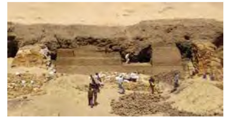
Fig.4 East enclosure wall showing the process of constructing the mud-brick foundation system (credits: Anthony Crosby, 2010)
