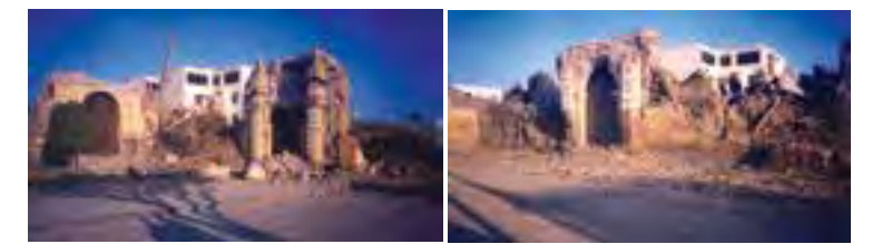
Fig.5 The Compañía Church, Pisco in 2007 after the earthquake: a) Area of the main façade and the entrance to the school, already separated from the rest of the wall pre-earthquake; b) Lateral façade also with separation cracks (credits: Pedro Hurtado Valdez, 2007)
