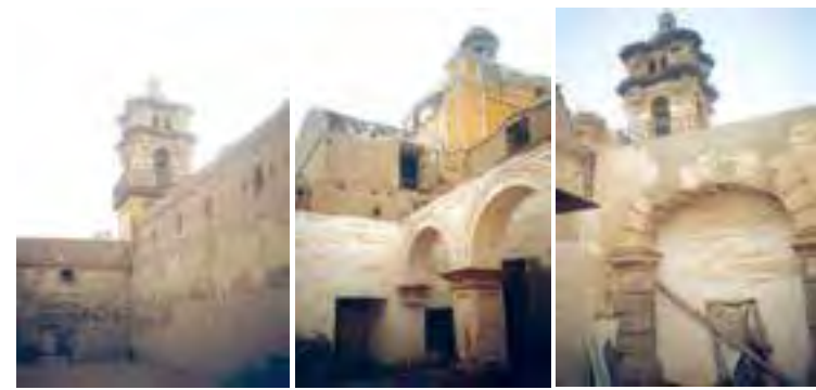
Fig.3 The Compañía Church, Pisco: a) Adobe walls coated with cement at the bottom; b) Earthen-framework vault and dome left weathering without an earthen coating; c) Adobe arch with cementitious-coating renovation (credits: Pedro Hurtado Valdez, 2007)
