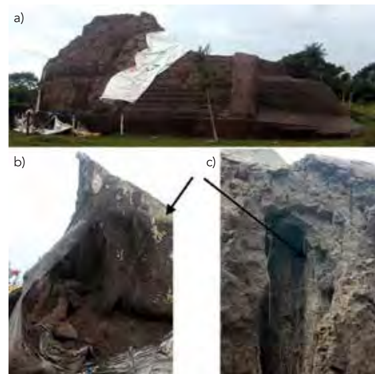
Fig.6 La Joya Pyramid in September 2010, after hurricane Karl: a. west façade with torn tarpaulins, southern sector (on the right) with polymer layer in good condition, b. collapse of north profile fill, arrows indicating weeds and roots, c. detail of weed roots in old crevices, originally filled with sand (credits: Annick Daneels, from project authorized by the Archaeology Council of Mexico's National Institute of Anthropology and History)
