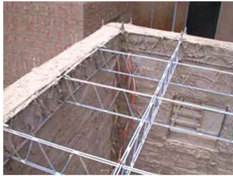
Fig.3 The unreinforced corner had no major complications. Note that the rack truss, which functions as the ceiling joists, also functions as a perimeter beam (credits: Adell, 2008)
