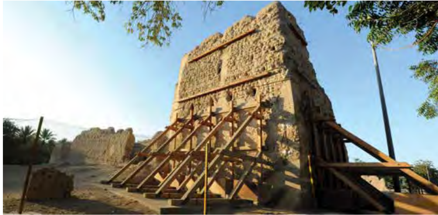
Fig.4 Abdullah Bin Salem Al-Darmaki House showing steel pinning and shoring (credits: Salman Muhammad © ADACH, 2011)
