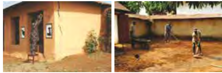
Fig.1 and fig.2 Preventive measures at the Royal Palaces of Abomey, 1996, Prema Project, ICCROM, CRAterre, DPC Benin (credits: Thierry Joffroy, 1996)
