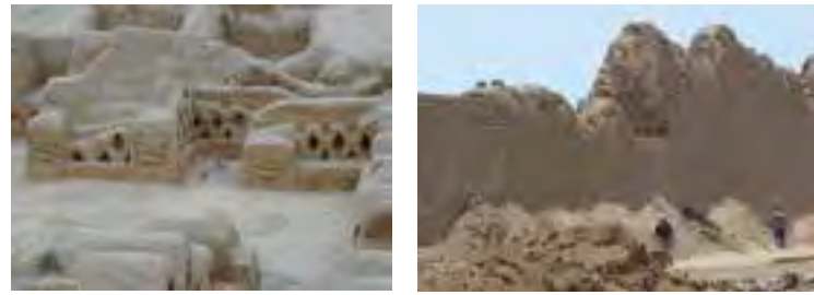
Fig.8 A sacrifice layer of gravel is used to protect the top of the walls. Audiences sector, Tschudi palace (credits: Mariana Correia, 2005) Fig.9 Reconstruction of the surrounding wall in Velarde palace, Chan Chan (credits: Luis Guerrero, 2007)
