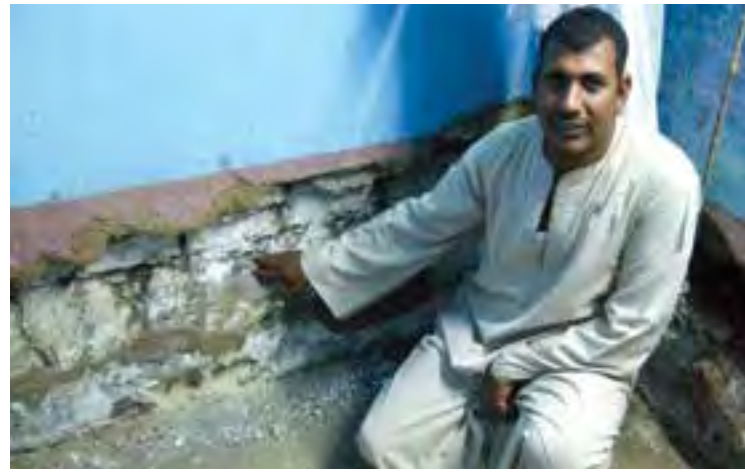
Fig.1 New Gournia Resident showing effects of rising damp (credits: World Monuments Fund/Community Consortium, 2010)
