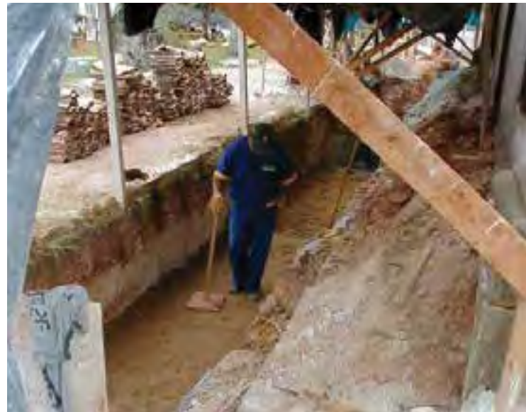
Fig.2 Rammed-earth veneer to protect the foundations of the Igreja Matriz De Santo Antonio (credits: Silvia Puccioni, 2000)
