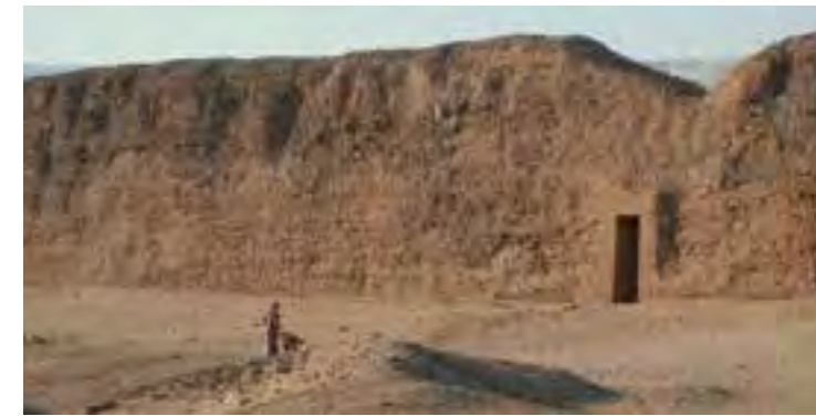
Fig.7 The west enclosure wall from the north after completion of the west gateway stabilization and restoration (credits: Anthony Crosby, 2010)
