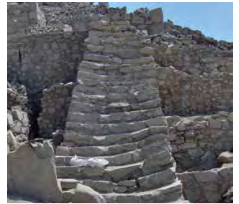
Fig.5 Unstable stairs requiring the renewal of shicras (credits: Julio Vargas, 2011)
