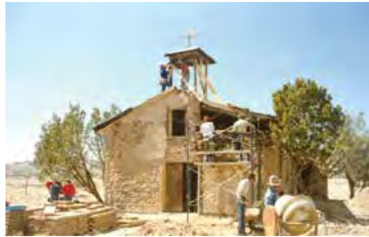
Fig.1 La Capilla de la Sagrada Familia at Pajarito, New Mexico during community-preservation efforts (credits: Ed Crocker, 1992)
