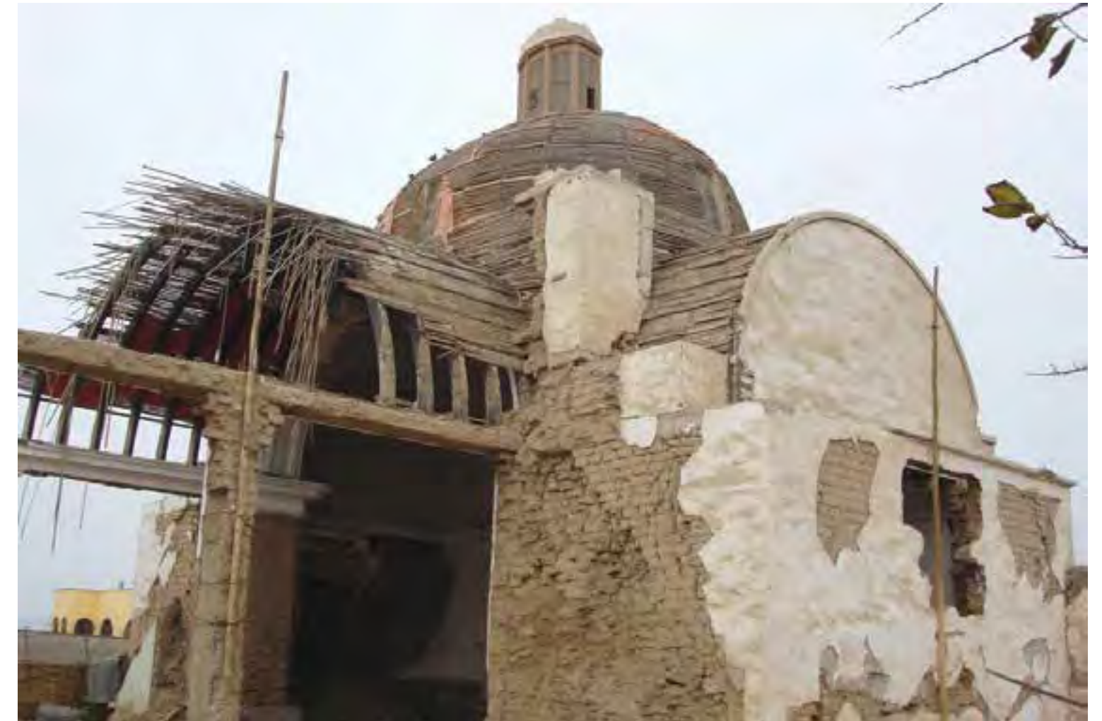
Fig.5 Avoid strengthening with reinforced concrete beams and columns, because they aid in collapse instead of protecting adobe walls, as in this example of the church of San Luis de Canete, damaged during the Pisco earthquake in 2007 (credits: J. Vargas-Neumann, 2007)
